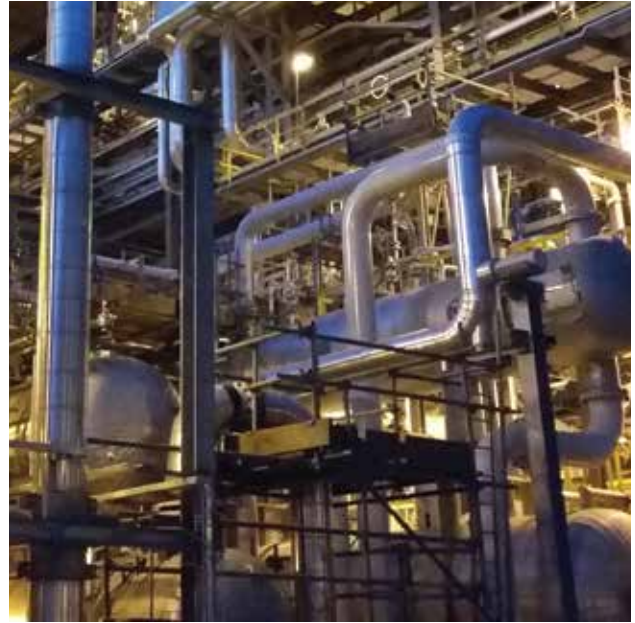
Industrial & Process Cooling Refrigeration
